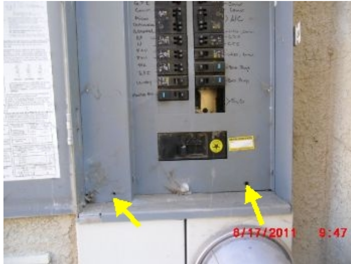
Panel cover screw(s) missing.
