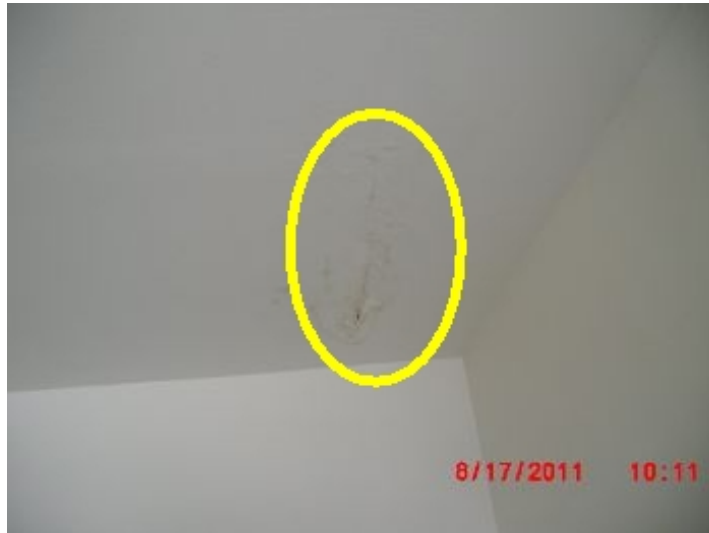
Water damage on ceiling below master bath-needs repair(2)
