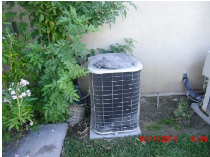
Upper level compressor did not operate(2)
