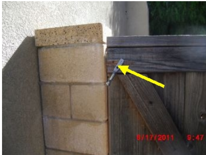
South gate latch loose*
